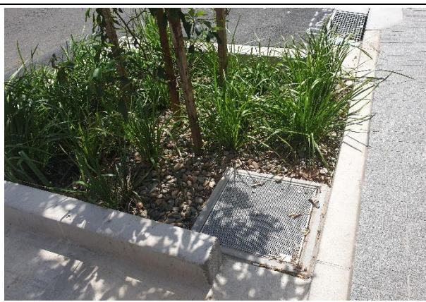
Tree pit installation with overflow pit in wrong location, as most runoff into the asset will go to the pit before the tree. (City of Hobsons Bay) Source: Wave Consulting Australia.
