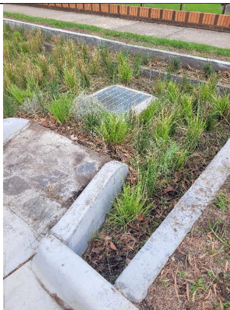
Raingarden installed in nature strip (Coburg, Merri-bek City Council). Source: Wave Consulting Australia.
