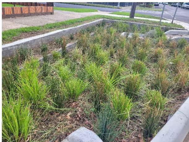
Raingarden installed in nature strip (Coburg, Merri-bek City Council). Source: Wave Consulting Australia.
