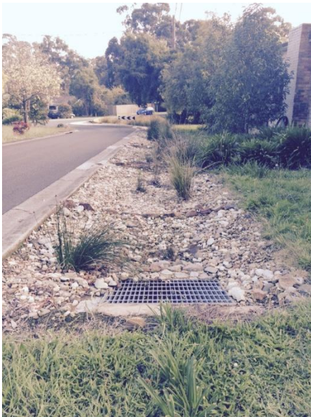
Simple rock lined swale (Mornington Peninsula). Source: Wave Consulting Australia.
