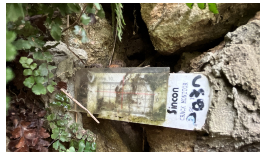
crack monitor between walls. Movement in two axis suggests sliding motion
