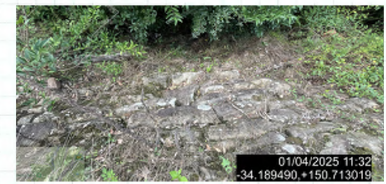
minor bulging around CH250
