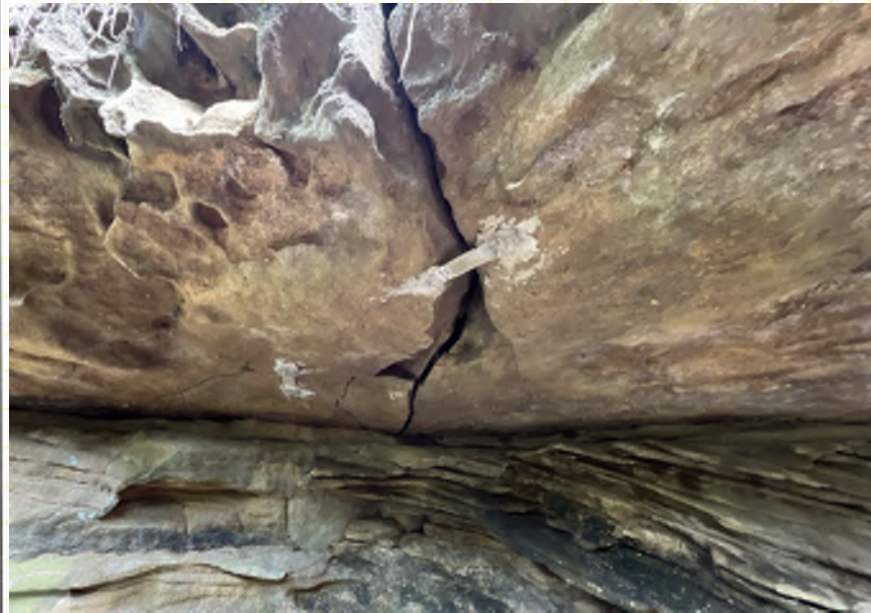
cracking in overhang
