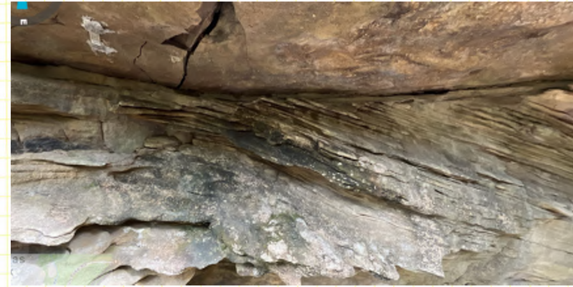
close bedding planes, with evidence of seepage
